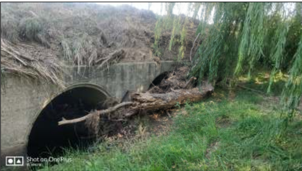
Culvert Aurville Road – upstream blockage
