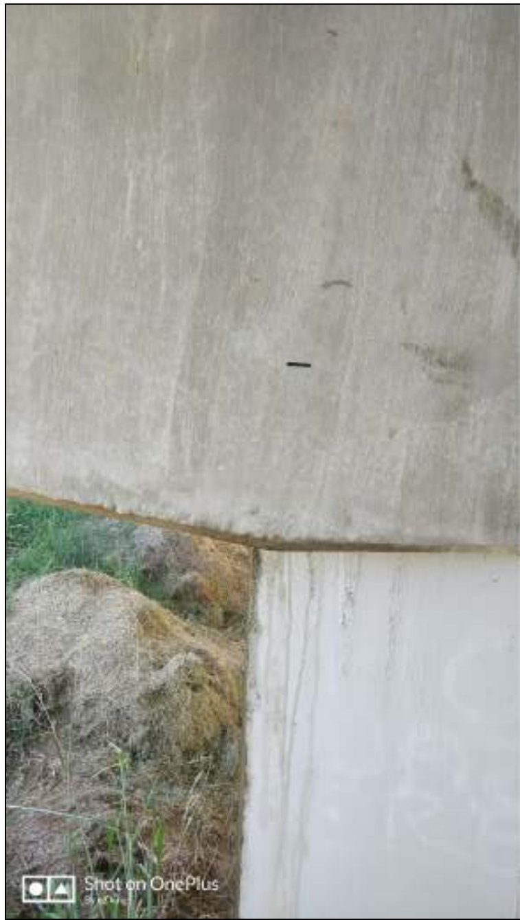
Flood Mark 1 – Close view
