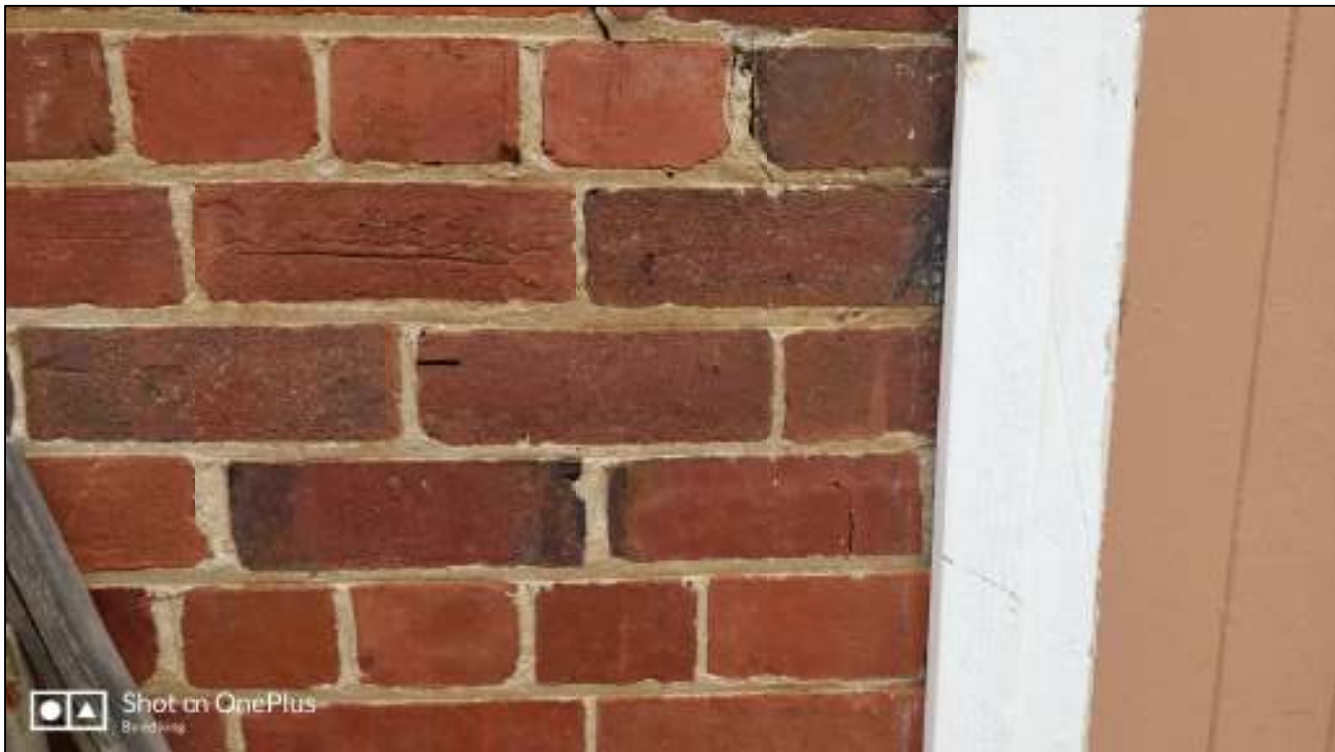
Flood Mark 2 – Close view
