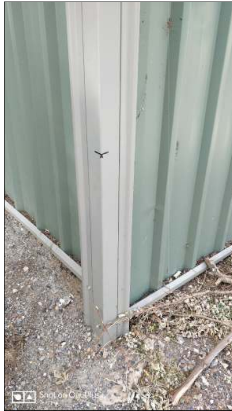
Flood Mark 3 – Close view
