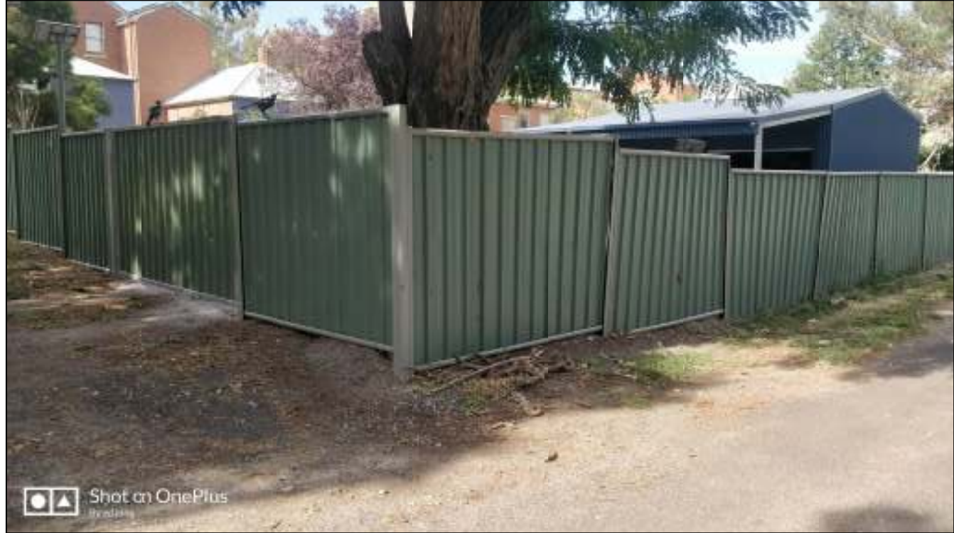
Flood Mark 3 – Corner of fence
