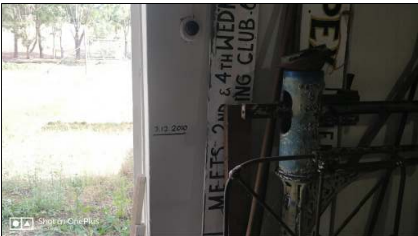
Flood Mark 2 – As marked on internal wall
